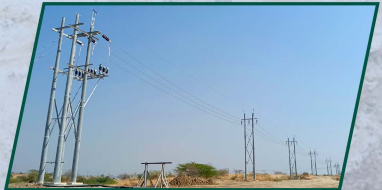
33KV TRANSMISSION LINE
